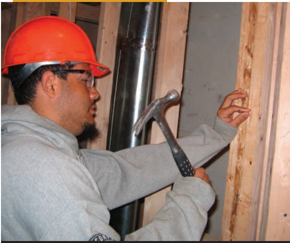
James Suarez helps to rehabilitate a house in Nicetown as part of his training in the construction program.
