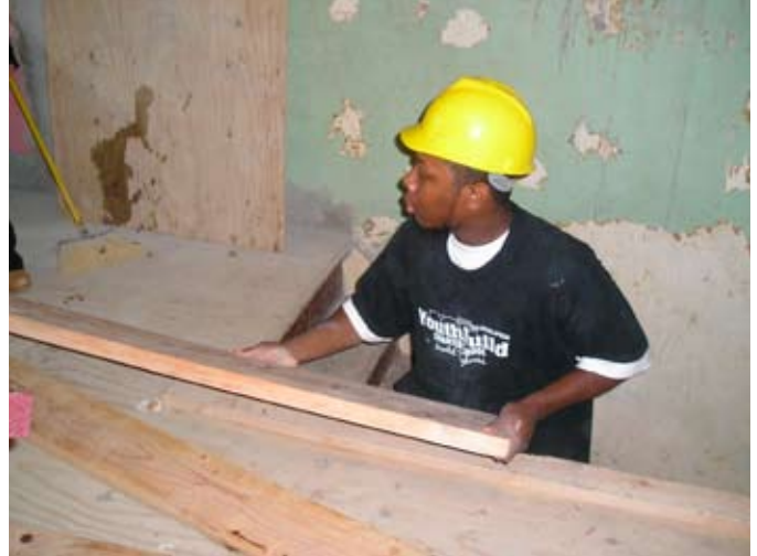
Construction student Shikeem Dorsey helps to build a home on North 26th Street. YouthBuild students rehabilitated the home over the course of the school year.
