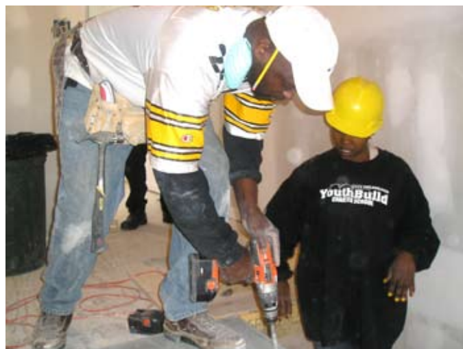
YouthBuild's funding sources make it possible for the school to provide valuable hands-on vocational training to approximately 215 students per year.
